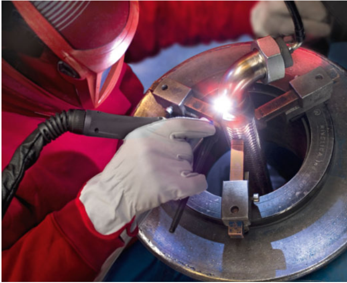
The work of the certified welders is accurate down to the millimeter or even the tenth of a millimeter.
